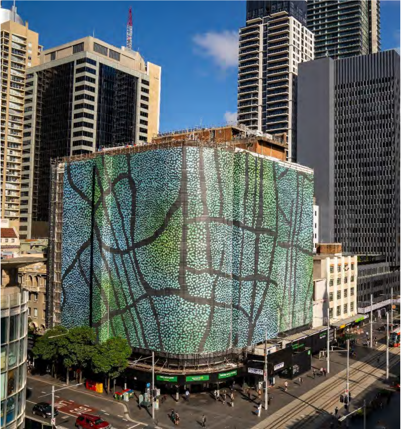
Figure 10. Creative hoardings covering the building, corner of Park and George Streets, during its 2022 renovation – Photo by Abril Felman / City of Sydney
