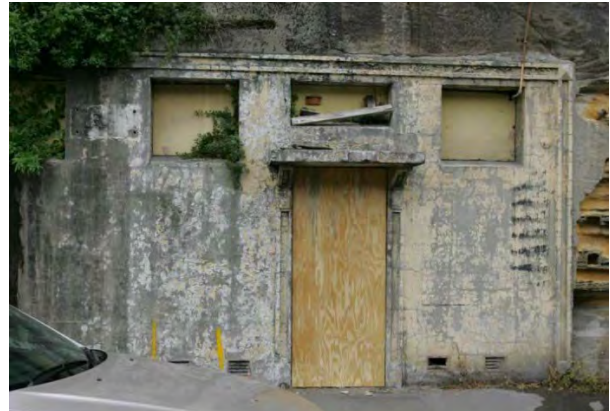
Condition 5 – Very Poor
