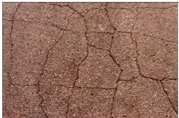
Condition 5 – Very Poor
